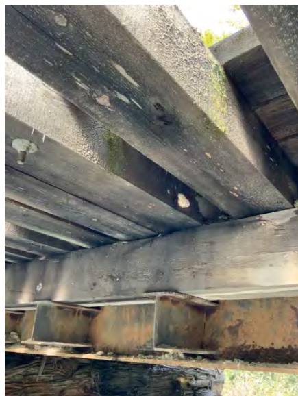
Ties starting to get fungus
