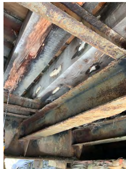
Ties starting to get fungus
